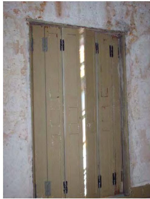
Shutters requiring restoration
